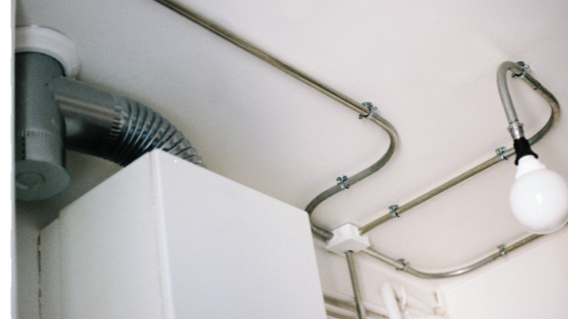
Electricity veins and exhaust gas arteries Paris, France (75)
